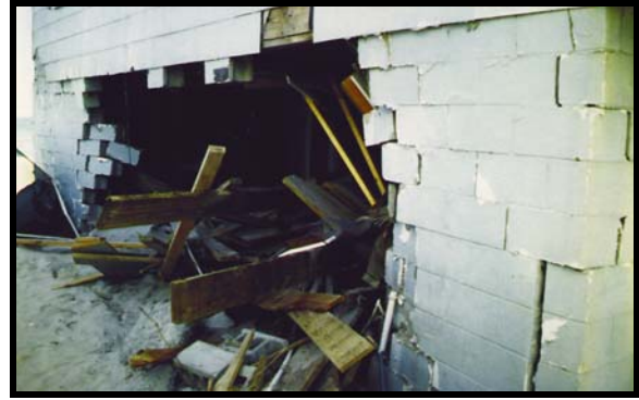
Figure 2-8. House damaged by high-velocity flows and debris loads.
