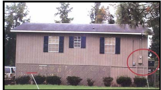
Figure 17-4. An example of restricting most of the enclosed lower area to latticework. Note the elevated electric meter and utilities.
