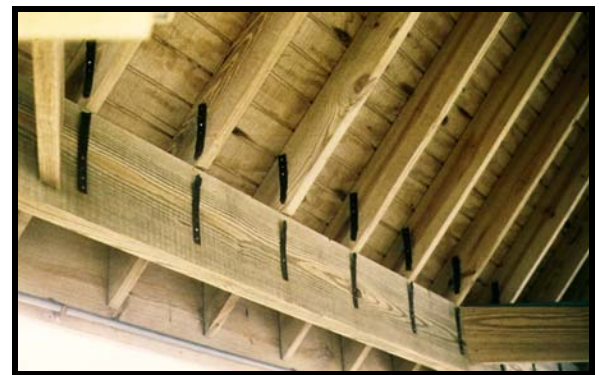
Figure 2-12. Hurricane straps rusted through by salt spray.
