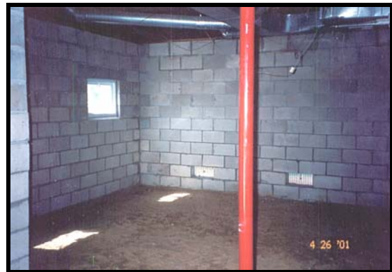
Figure 11-9. This is how an enclosure below an elevated building should look, but over time the owner may want to improve and finish the area.
