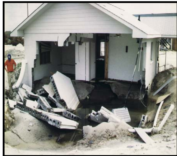
Figure 2-9. Localized scour undermined this slab-on-grade house on the coast.
