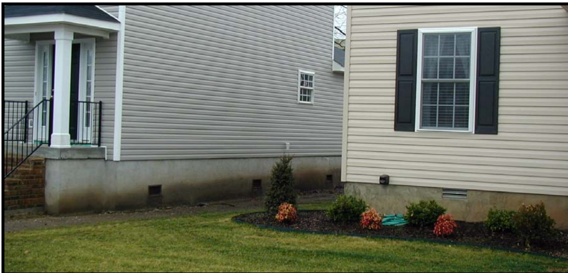
Figure 11-8. The house on the left has compliant crawlspace openings. The openings in the foundation on the right are too high.
