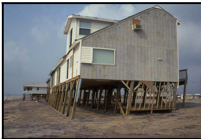
Figure 16-5. This house had inadequate pile embedment and cross bracing.
