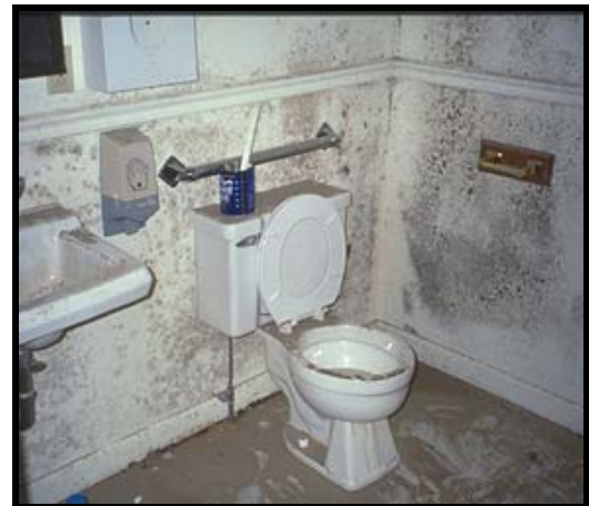
Figure 2-6. Post-flood silt, mold, and mildew.
