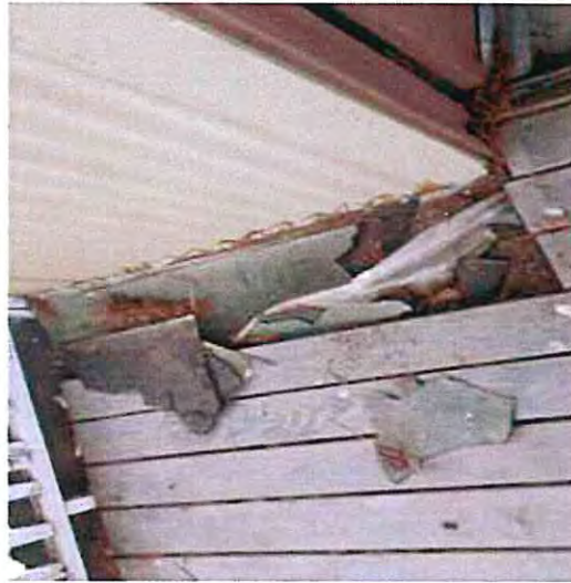
Photograph No. 12 View of roofing shingles with tar on second floor balcony.
