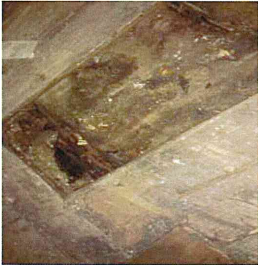
Photograph No. 9 View of brown vapor barrier below wood flooring on first floor.
