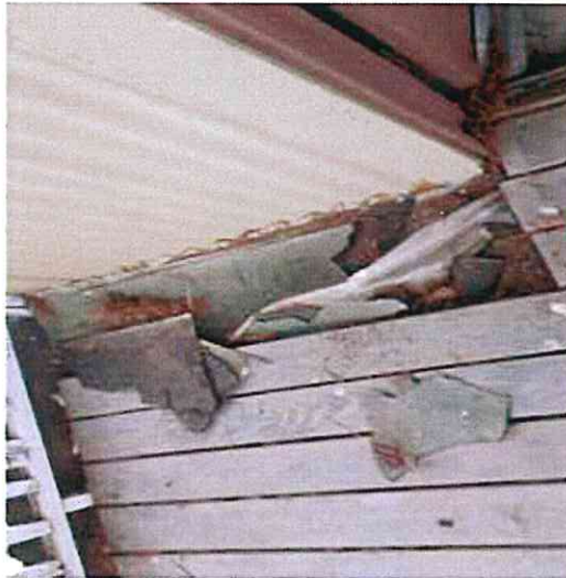
Photograph No. 12 View of roofing shingles with tar on second floor balcony.
