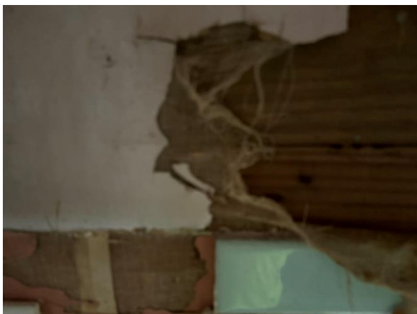
Photo #5: View of HA-5 – 2x4 Light blue bathroom tile with associated thin set/grout
