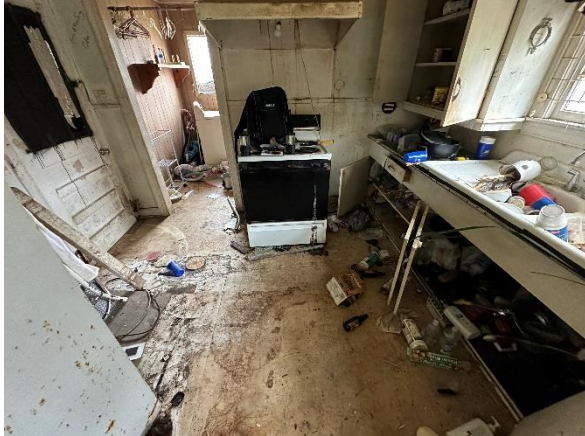
Photo #1: View of HA-1 - 12x12 White or Beige floor tile with associated mastic
