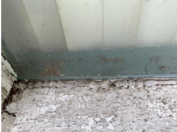
Photo #7: View of HA-7 – White exterior caulking along windows
