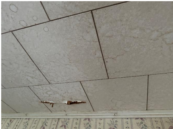
Photo #3: View of HA-3 – 12x12 white ceiling tile (stapled)
