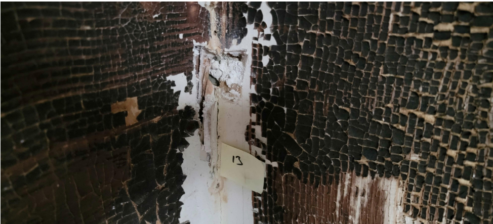
Photograph No. 11 HA-13: White Wallboard with Joint Compound and Tape
