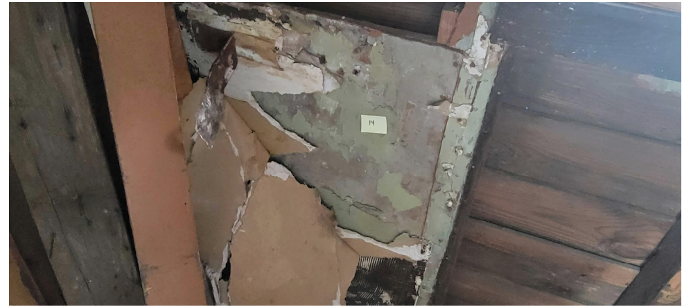
Photograph No. 12 HA-14: Green Water Barrier Behind Wallboard
