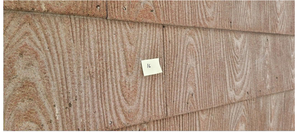
Photograph No. 14 HA-16: Brown Exterior Siding
