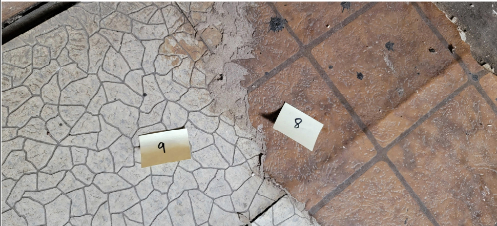
Photograph No. 7 HA-08: Brown Vinyl Sheet Flooring with Fibrous Backing & HA-09: White Vinyl Sheet Flooring with Black Mastic
