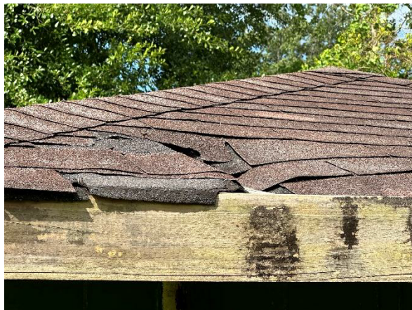
Photo #15: HA-15: Black roofing shingles and felt paper associated with detached shed
