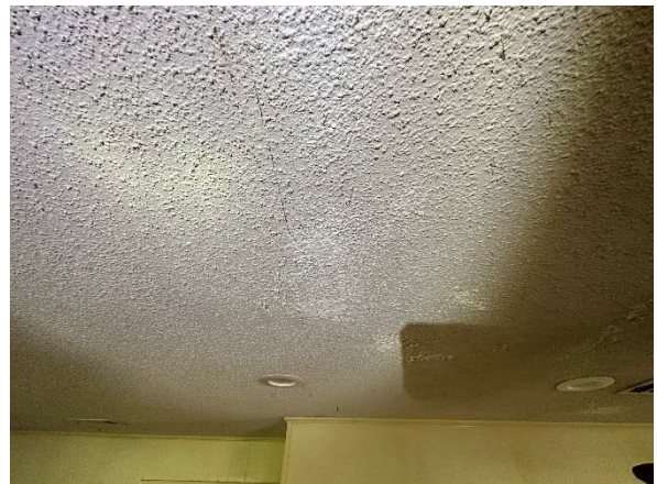
Photo #6: HA-6: White popcorn ceiling
